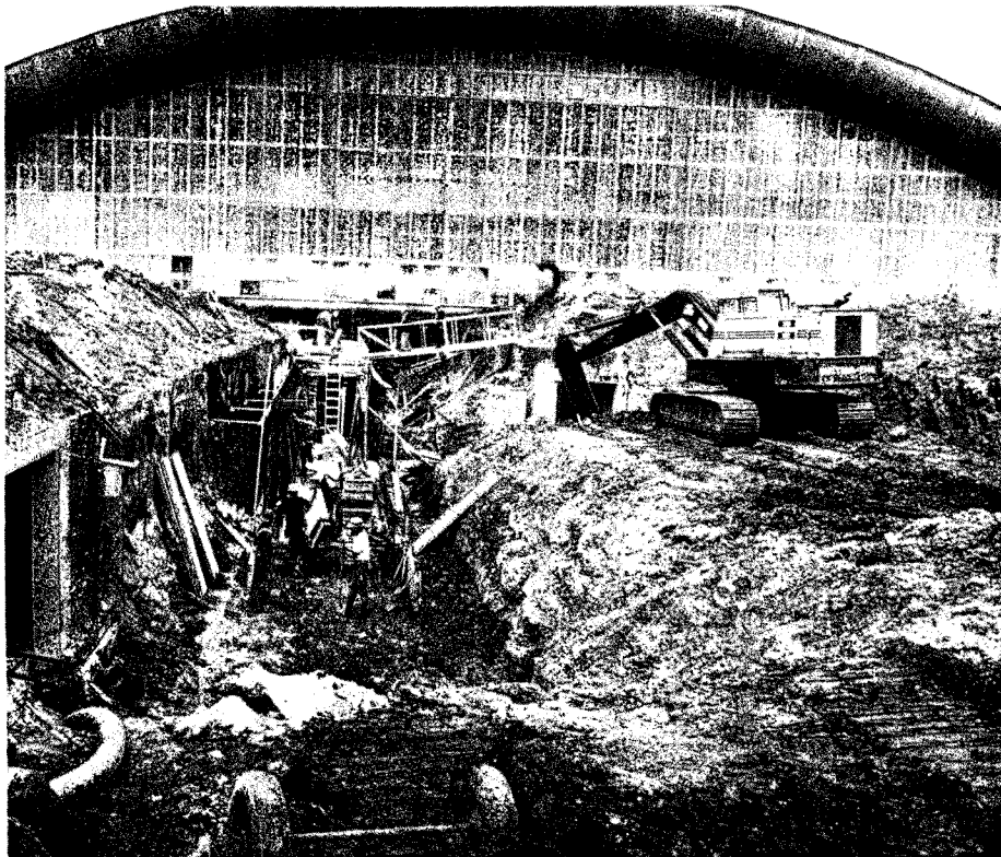
Drastic changes in the Fermilab landscape. For the Tevatron, the big Meson Experimental Hall becomes a Target Hall. New primary beam focusing enclosures are seen here under construction upstream of the hall. New experimental halls will be built downstream.
